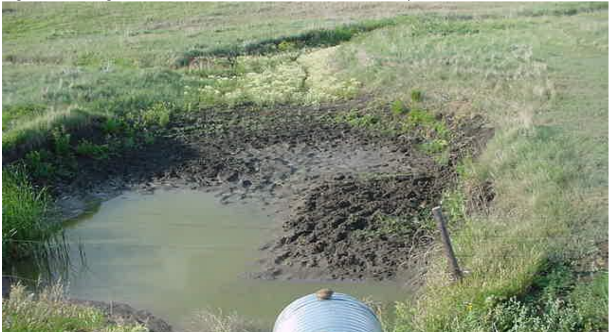
Figure 3. Weak Presence of Water: This stream only has a small pool of water in the scour hole below the culvert.
